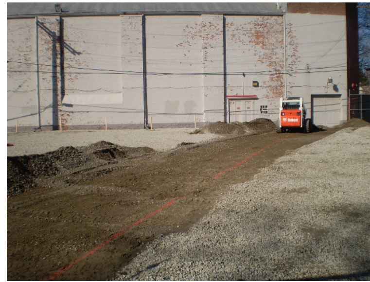
The line is drawn on the ground. Now to use the trenching machine to dig along the line.
