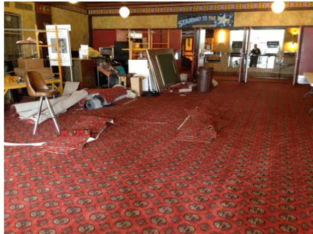
Left: Concession stand area nearing completion. Right: Outer lobby still has lots to do to finish up!
